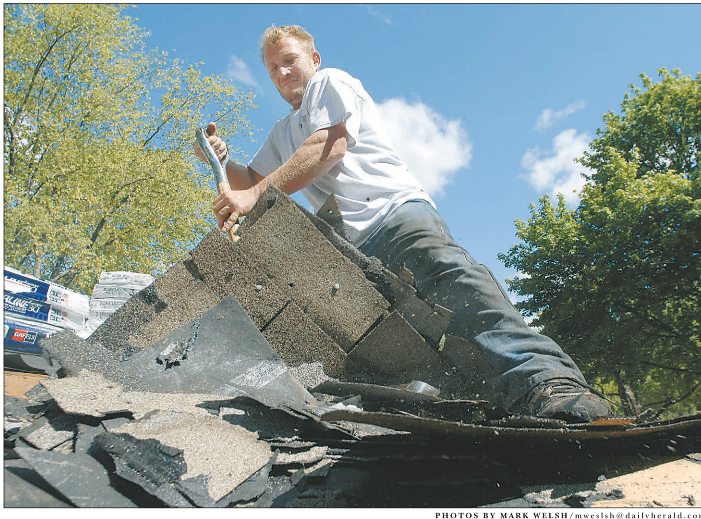
Using a pitchfork, Peterson Roofing worker Darek Andruszkiewicz, tears up a section of the roof of a home in Arlington Heights.
