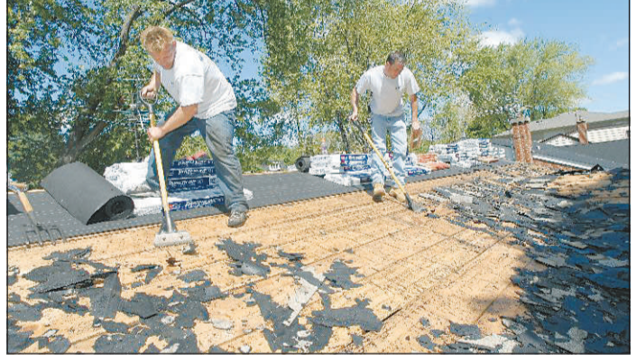
Mike Chrouser of Peterson Roofing, right, works with Darek Andruszkiewicz to remove old shingles and other materials before tacking down the new roof.
